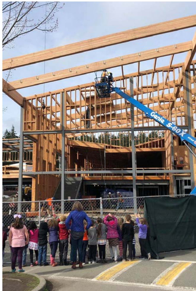
Salish Coast Elementary School phased construction presented a learning opportunity as children remained on-site throughout the process
